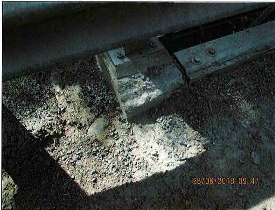
Localized spalls on Southeast ballast wall
