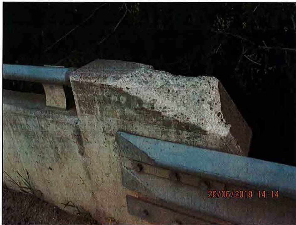
Spall at Northwest
