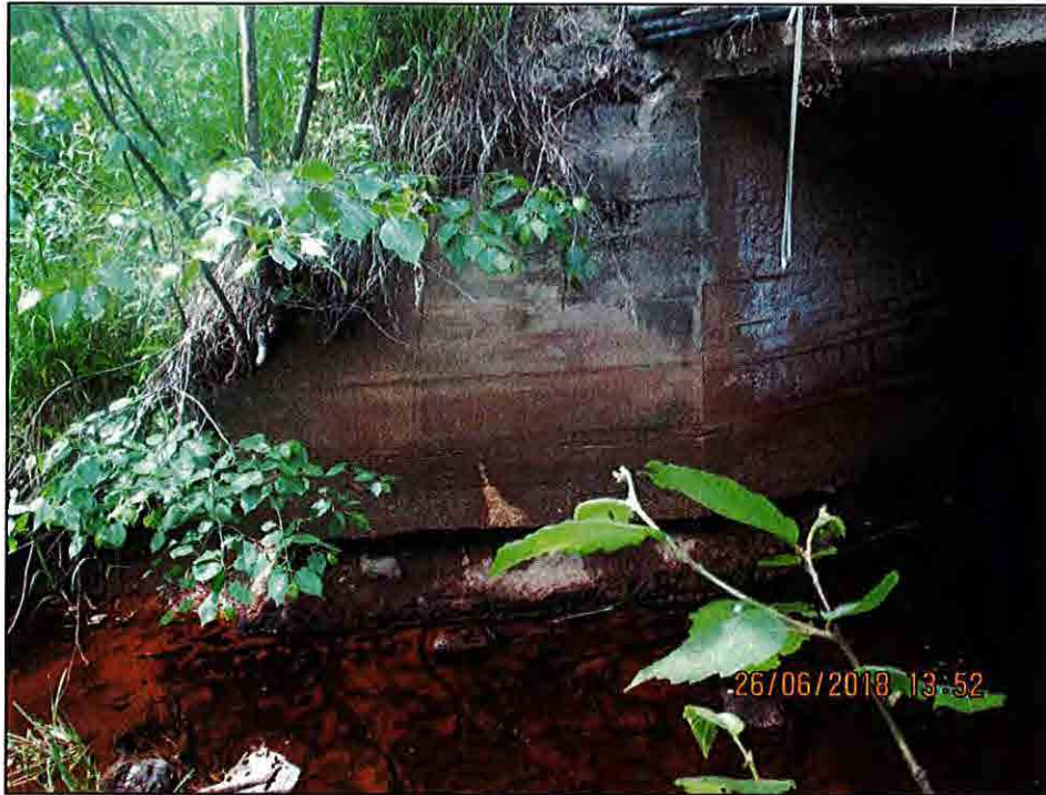
Severe undermining and scouring at Southwest wing wall
