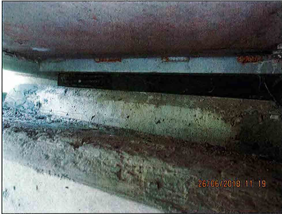
Northeast bearing – minor loss of contact of bearing (Typ. Southeast, Southwest, Northwest)
