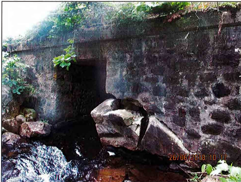
Partial failure at Northeast wing wall
