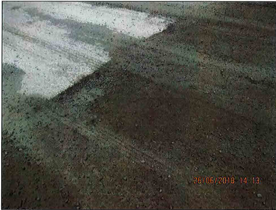
Potholes at South approach
