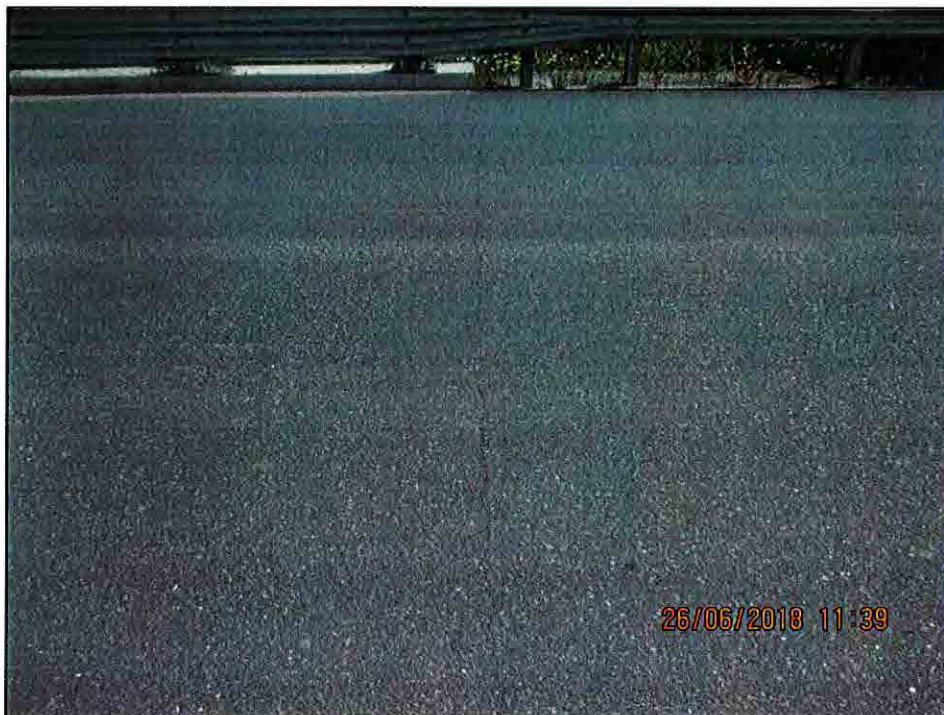
Narrow crack on South approach
