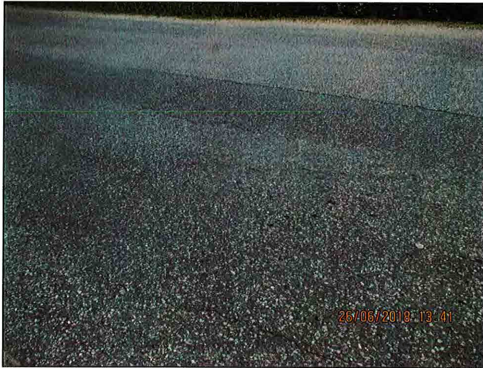
Cracks on wearing surface
