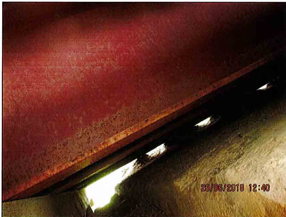
Corrosion of bottom flange
