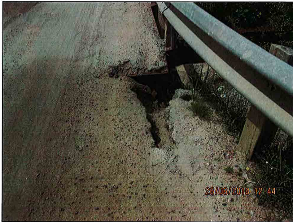
Localized severe erosion of the embankment and loss of material at Northeast
