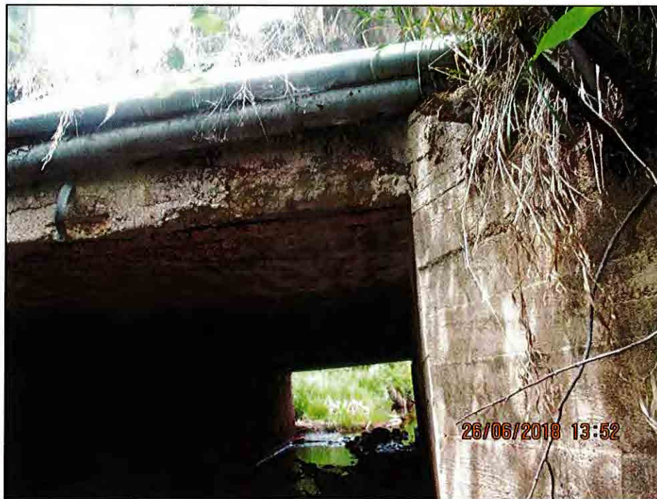
Severe spall at soffit (South end)
