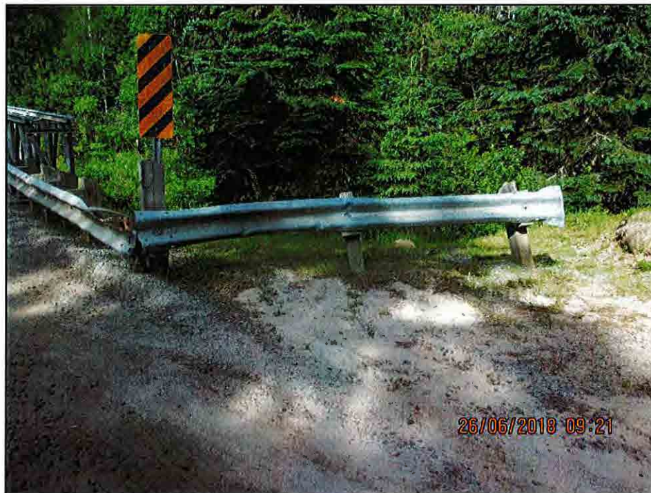
Damaged guide rail at Northeast
