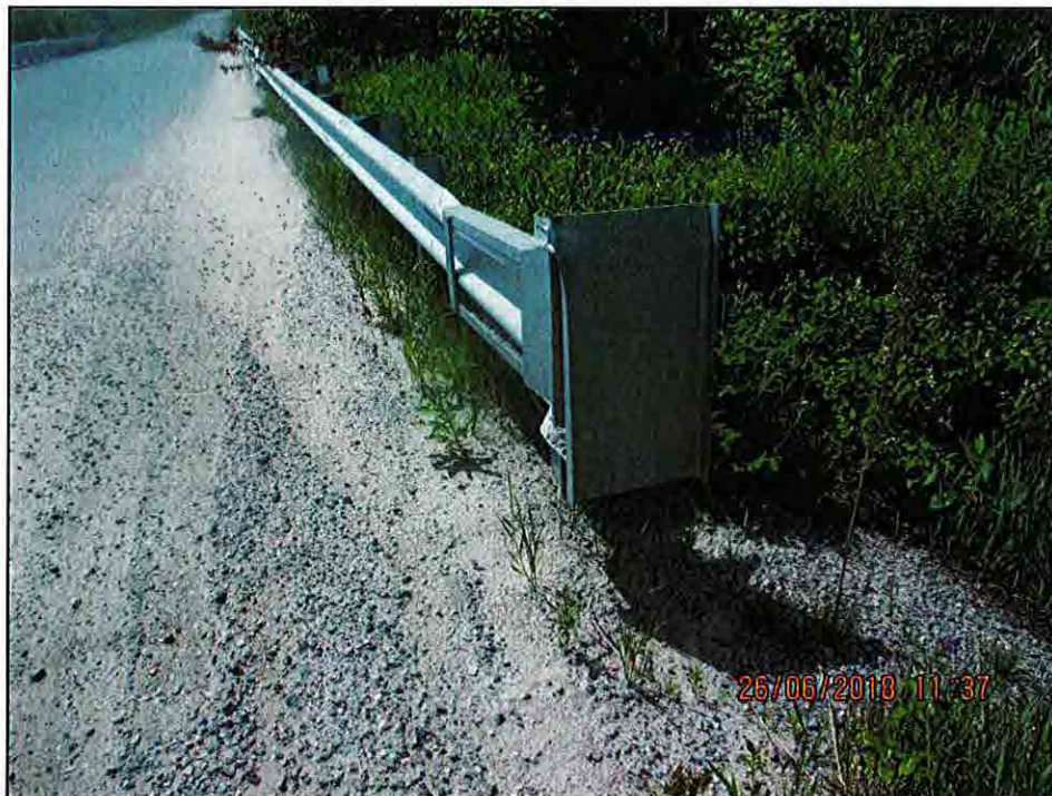
Minor damage at Northeast
