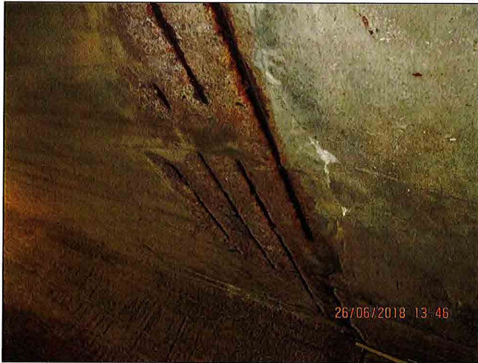
Spall at soffit
