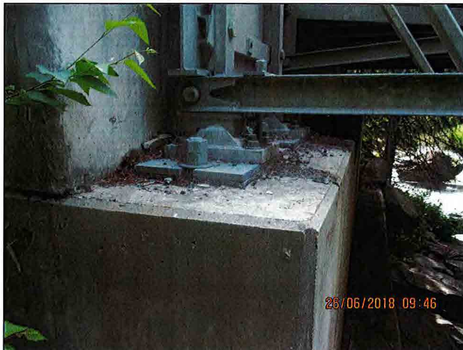
Debris at bearings (Typ.)
