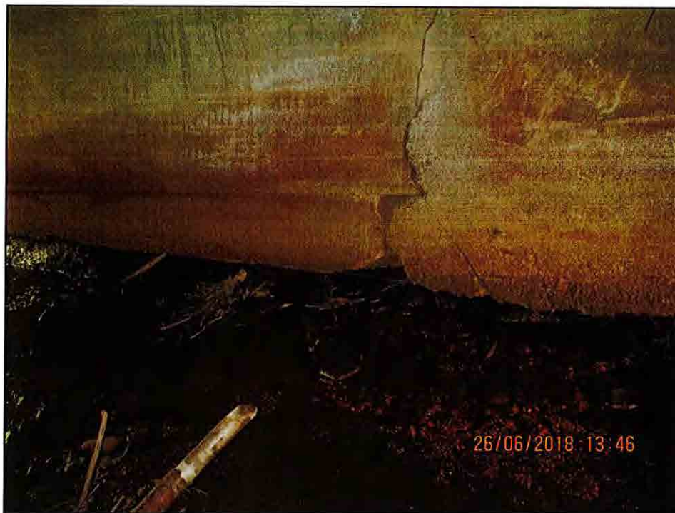
Concrete disintegration of abutment wall
