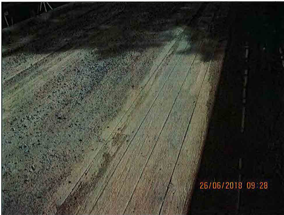
Rotting and splitting of wearing surface
