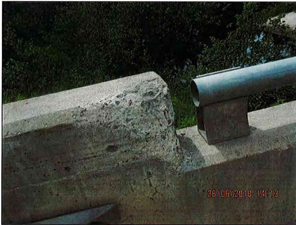
Spall at Southwest
