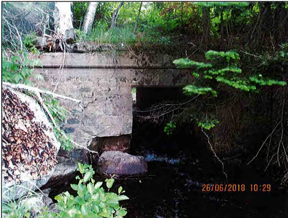
Partial failure of Northeast wing wall
