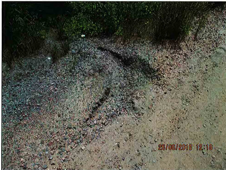
Minor erosion of embankment at Southeast
