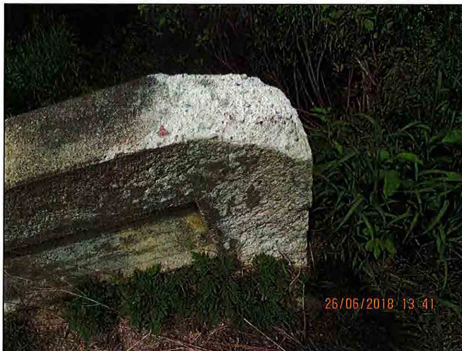
Spall at Northeast
