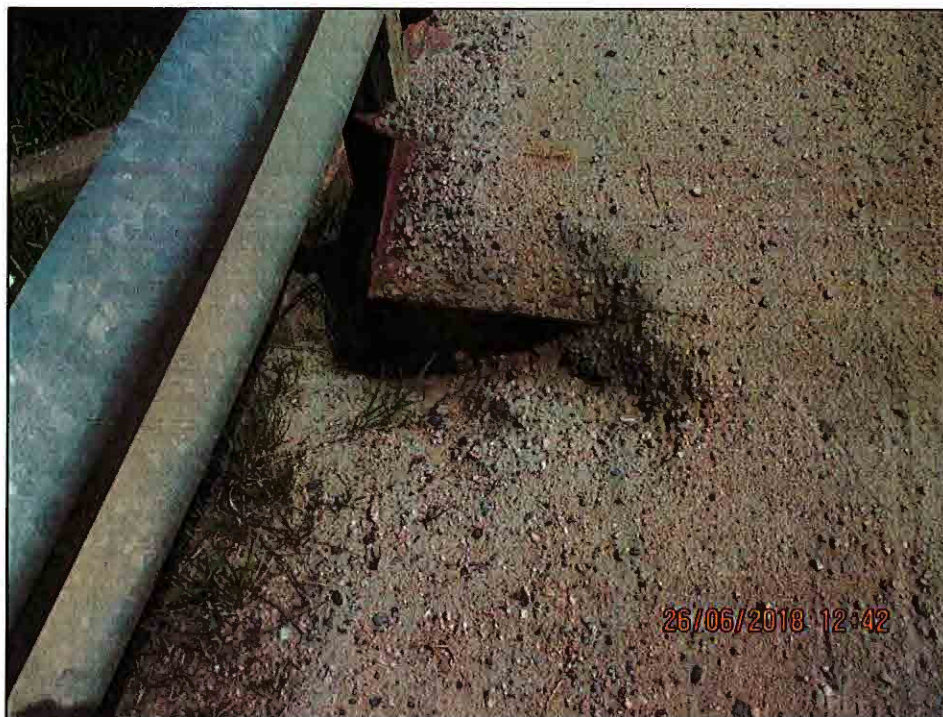
Localized severe erosion of the embankment and loss of material at Northwest
