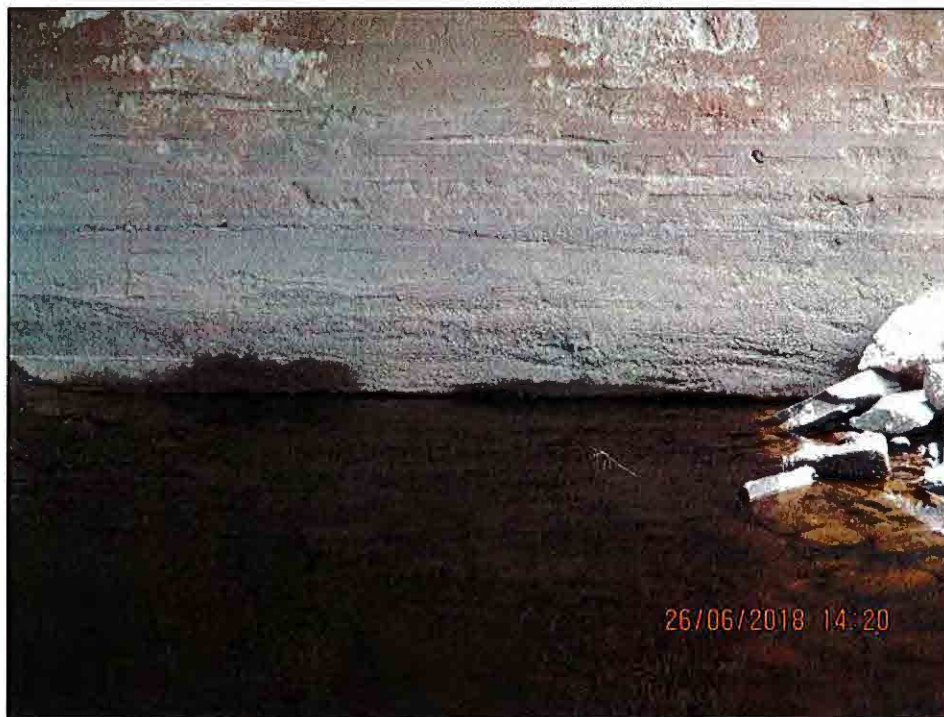
Undermining of South abutment
