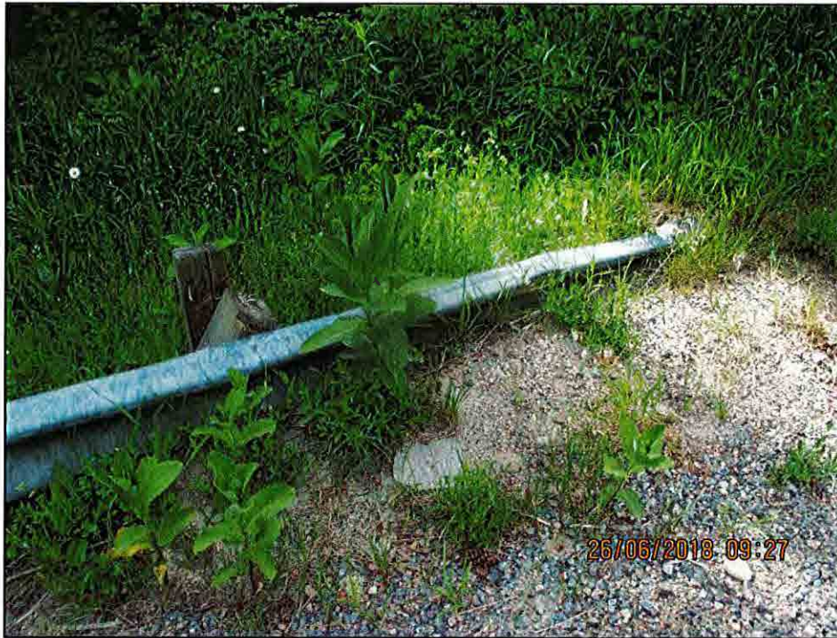
Damaged guide rail at Southwest
