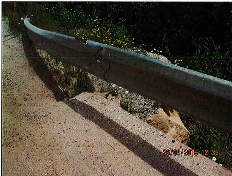
South railing – damaged posts
