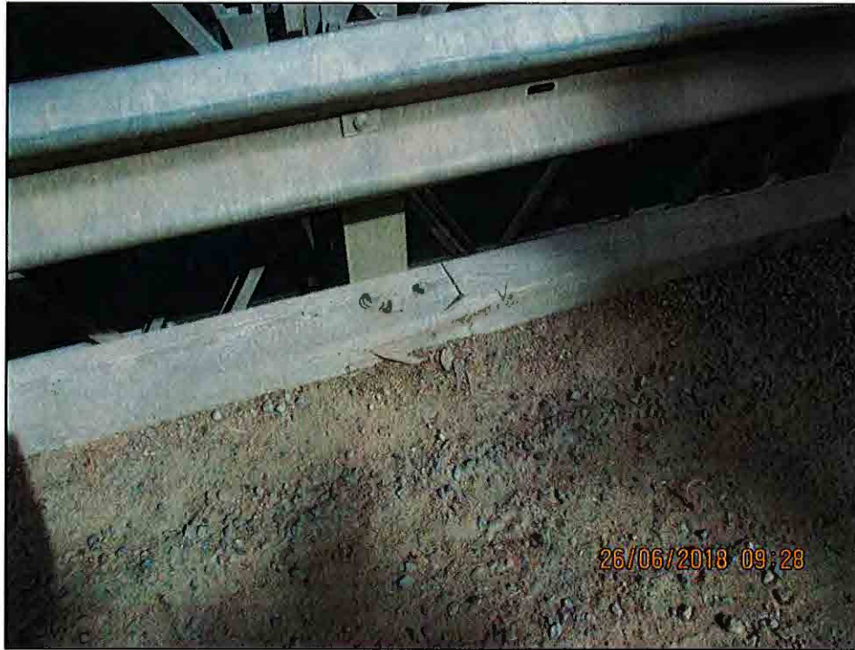
Damaged curb (North side)
