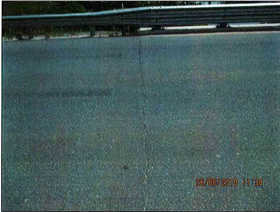
Medium transverse crack on North approach
