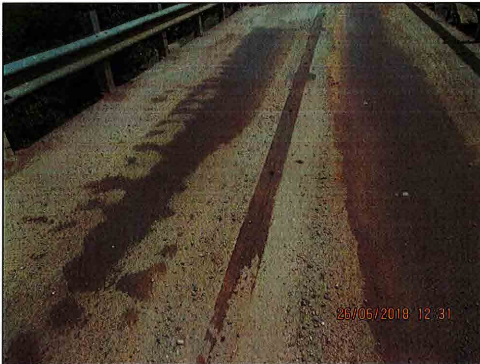
Debris on deck
