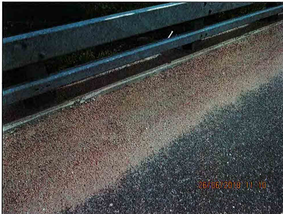
Accumulated sand on road
