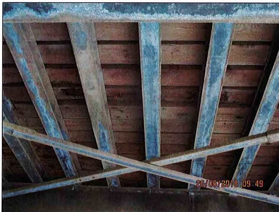
Moisture and rotting of soffit
