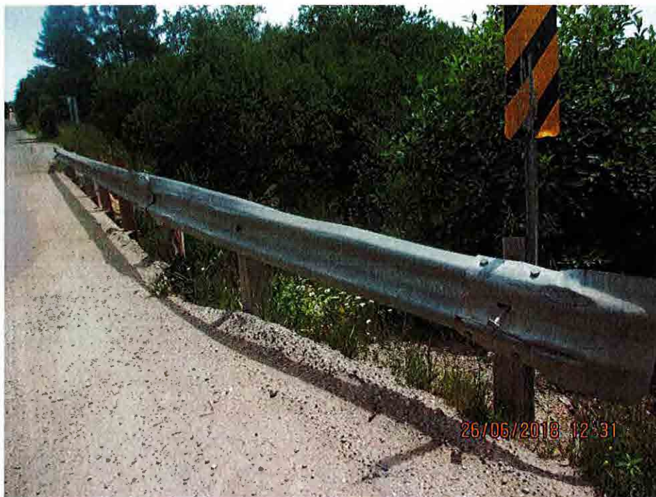
Severely damaged South railing
