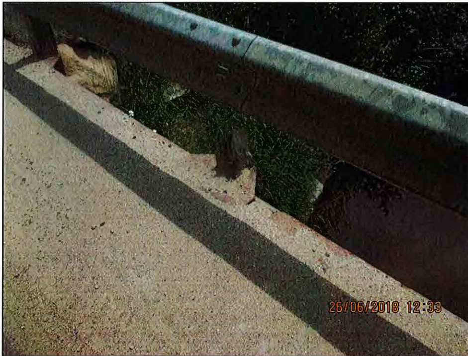
South railing – damaged posts
