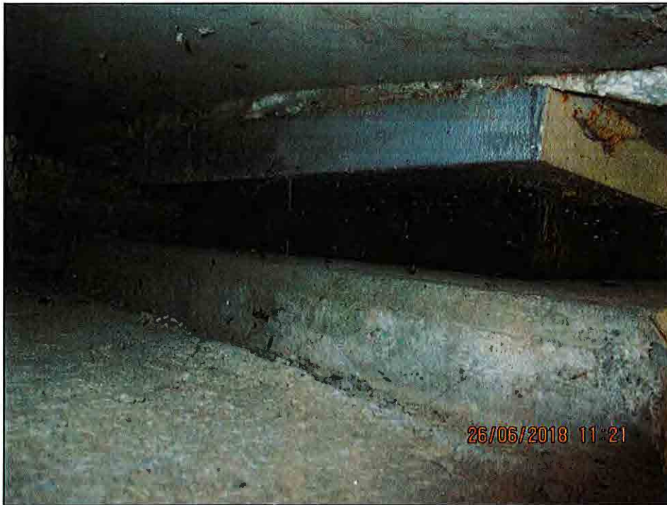
Minor loss of bearing contact
