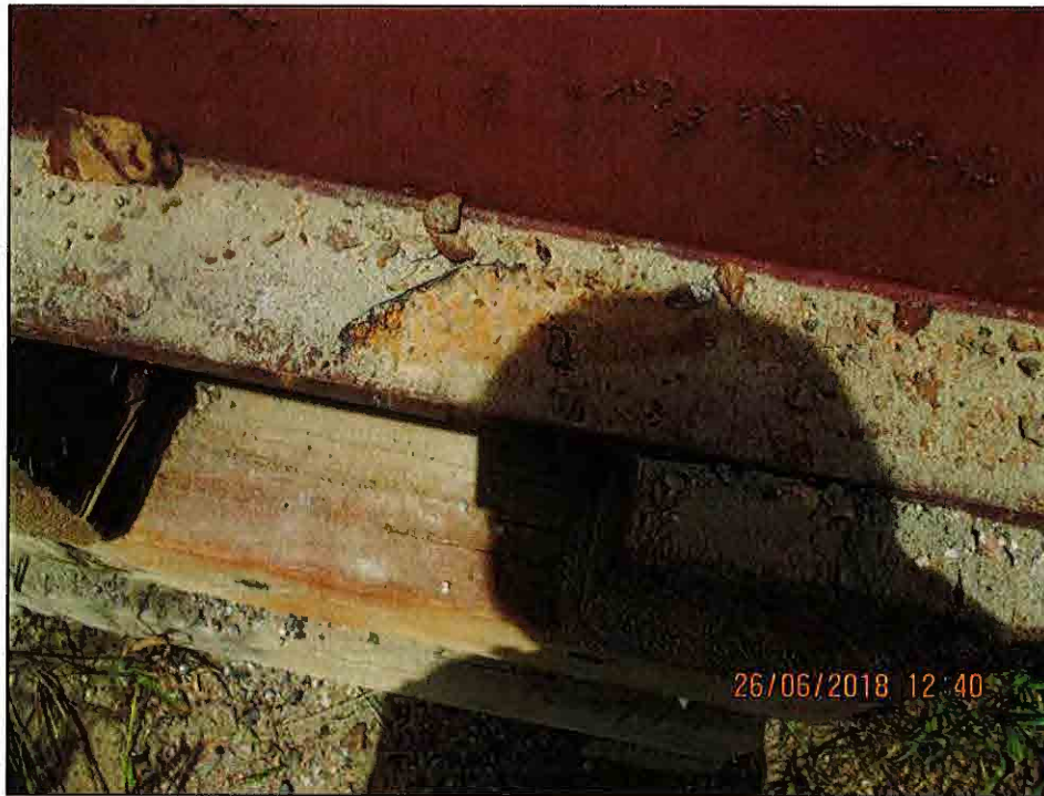
Flaking of exterior girder
