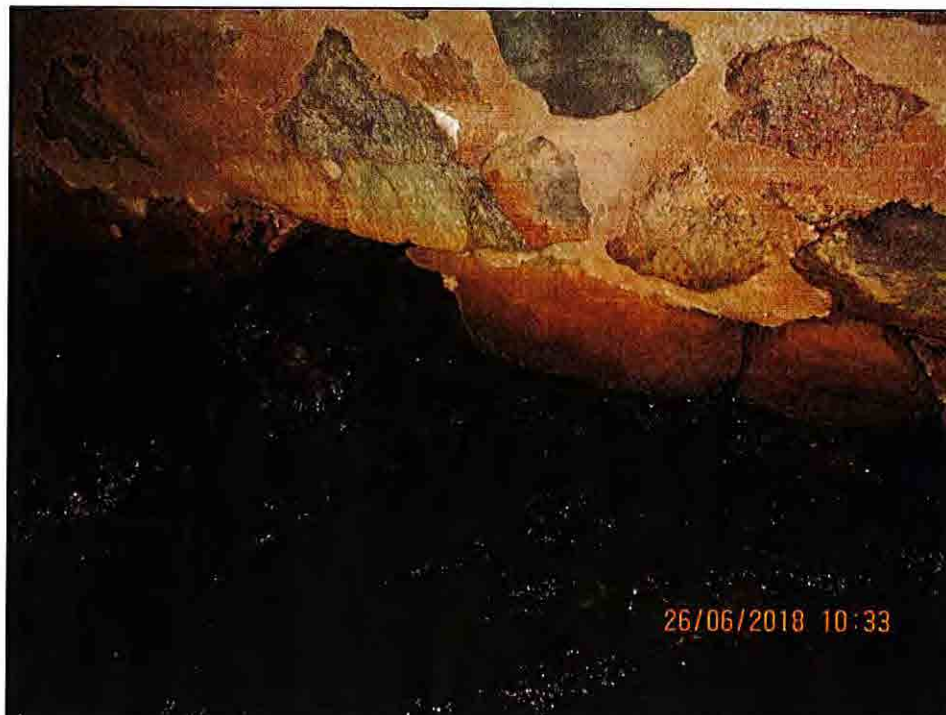
Scouring along the abutment walls
