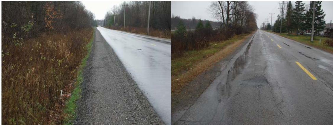
Figure 9 Steep Side Slopes -to be avoided in new construction
