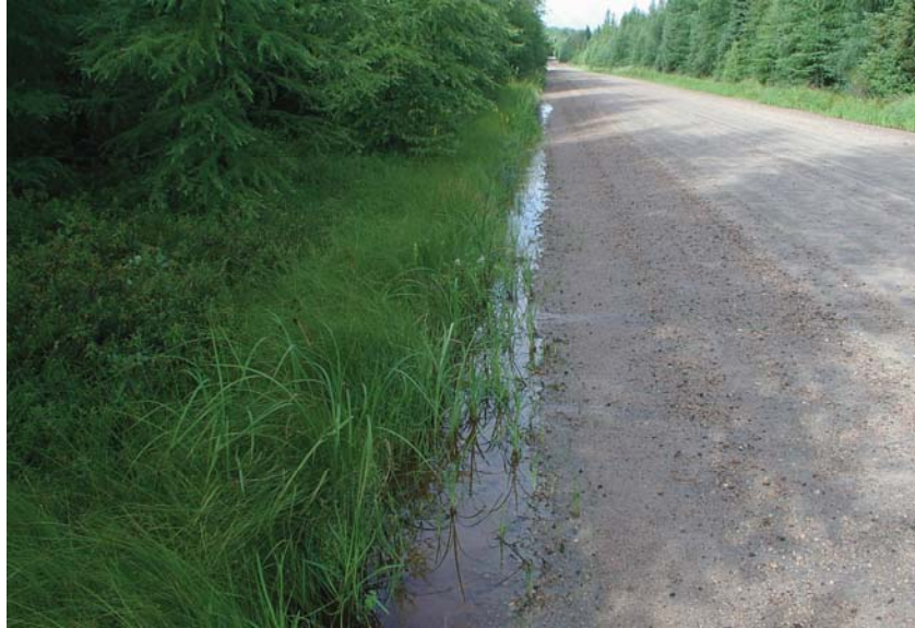
Figure 8 Inadequate Roadside Drainage
