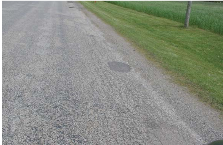
Figure 10 Shoulder Berm contributing to edge failure
