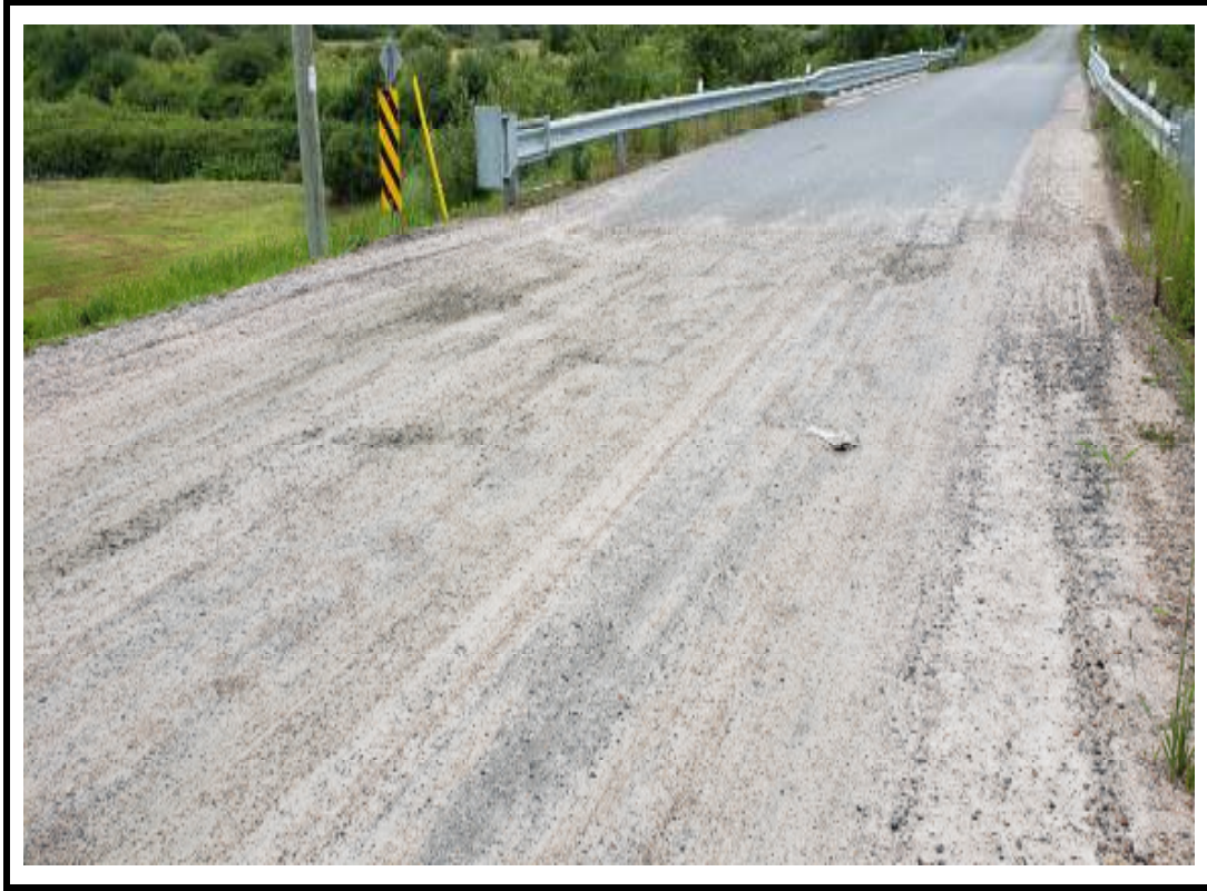
Photo 7 Potholes and loose gravel noted on approach wearing surface
