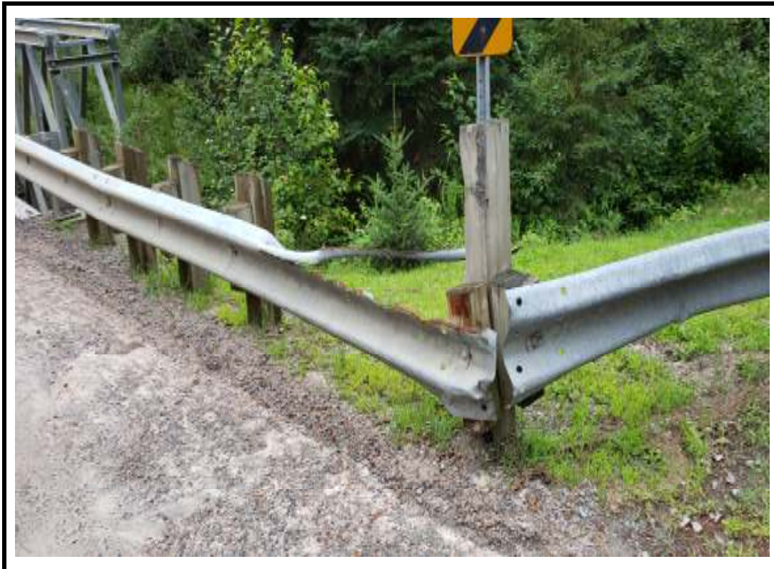
Photo 10 Damage with corrosion noted on thrie steel beam on northeast approach barrier
