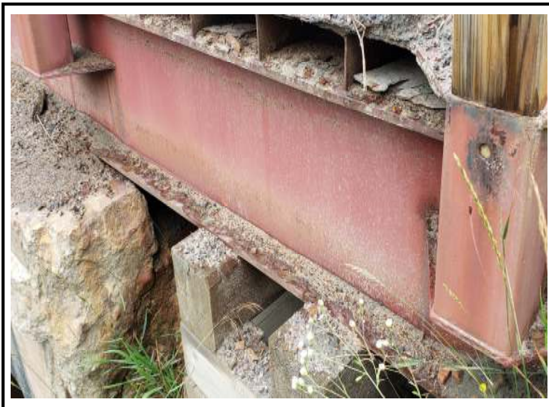
Photo 14 Moderate corrosion with pitting of coating noted on exterior beams at southeast corner
