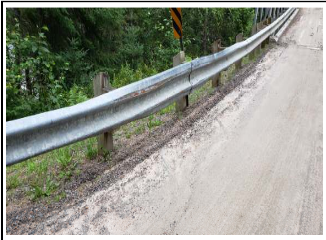
Photo 8 Collision damage observed on southeast approach barrier
