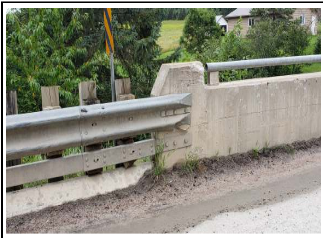
Photo 10 Collision damage noted at connection between approach and deck barrier
