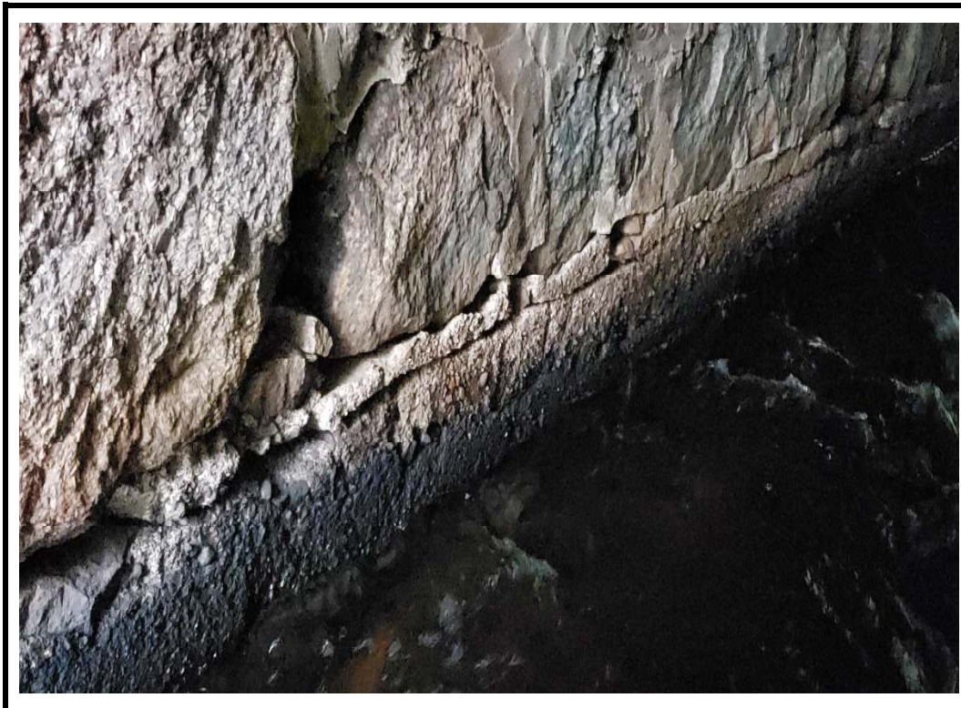
Photo 10 Moderate honey combing noted at base of abutment wall along waterline (prior to 2020 rehabilitation)
