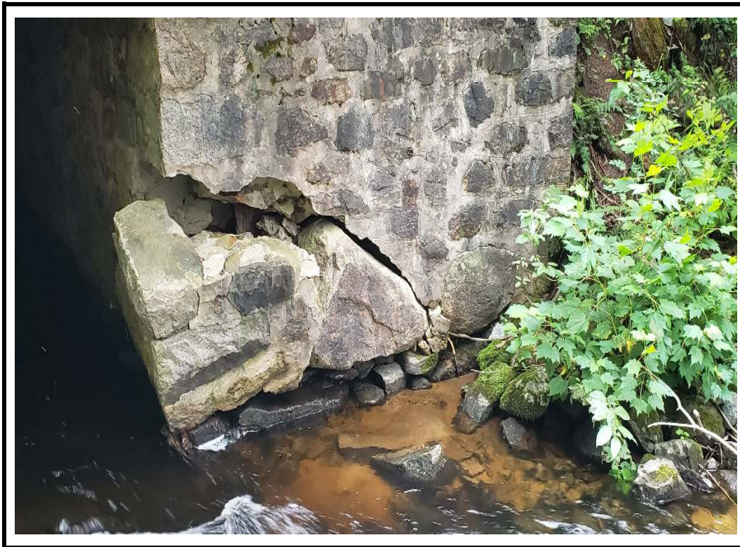
Photo 8 Large spall with disconnected portion noted at interface of north abutment wall and wingwall (prior to 2020 rehabilitation)
