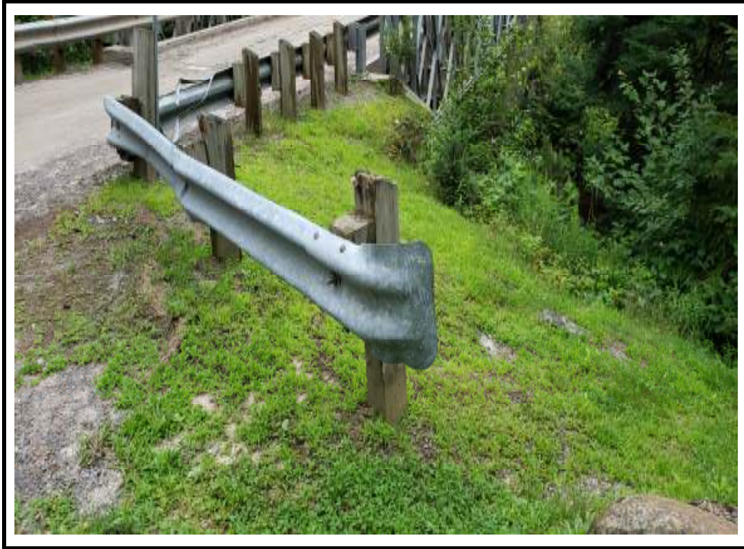
Photo 9 Substandard end treatment with damaged approach barrier at northeast corner
