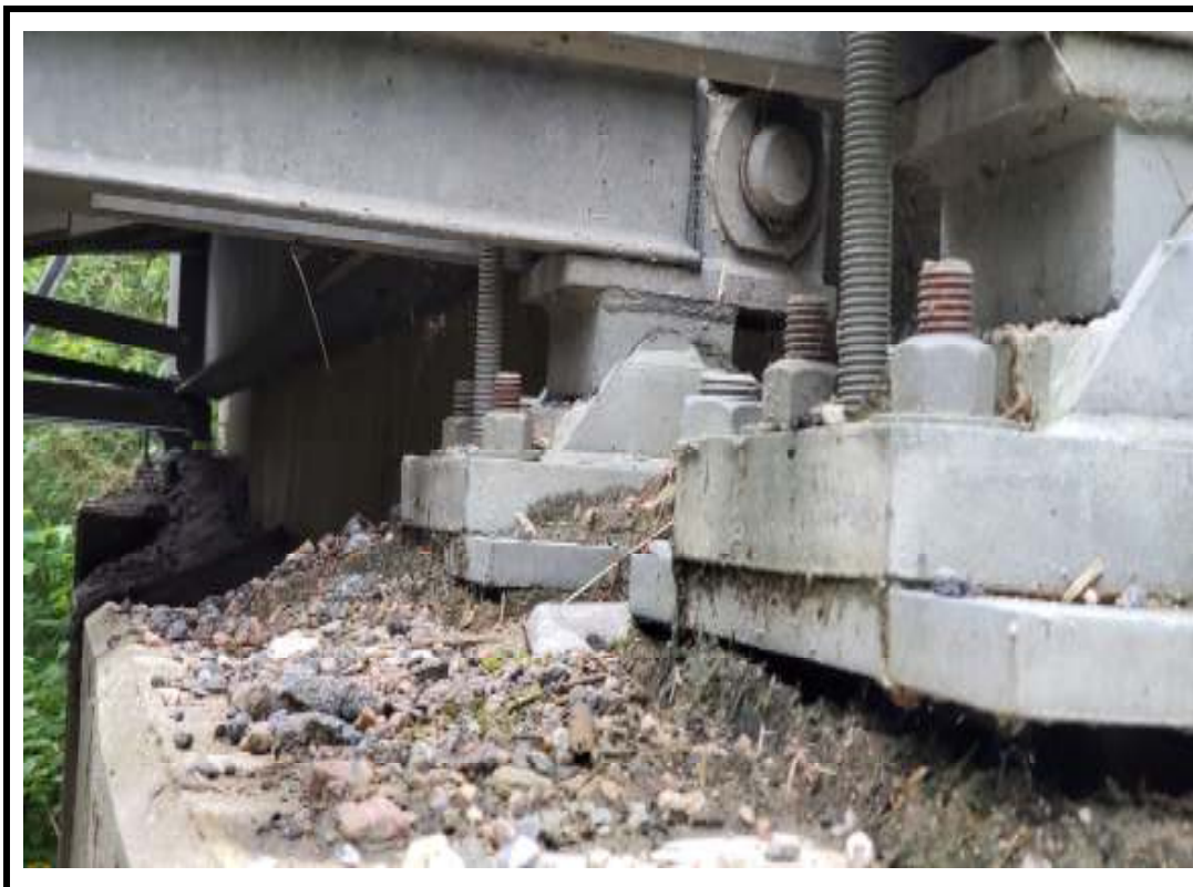
Photo 14 Debris accumulation observed around bearing pad
