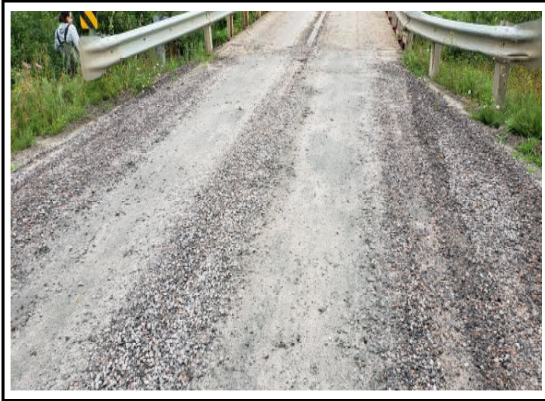
Photo 7 Loose gravel and potholes noted on wearing surface
