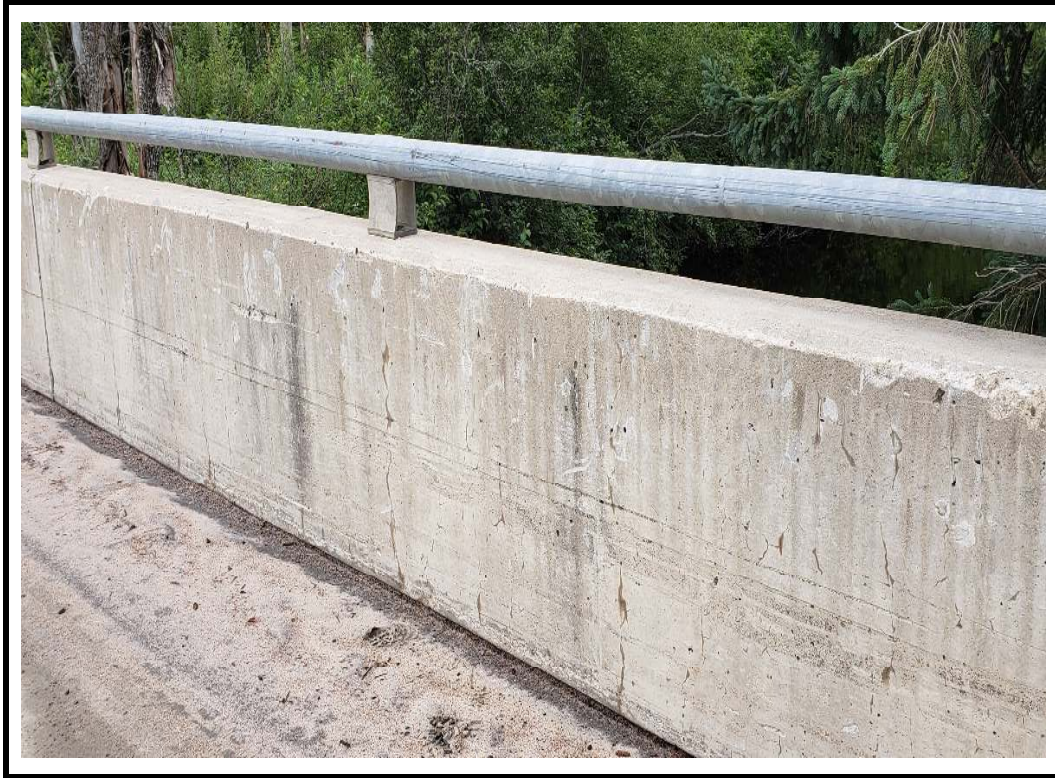
Photo 11 Narrow cracks with damp stains noted on parapet wall
