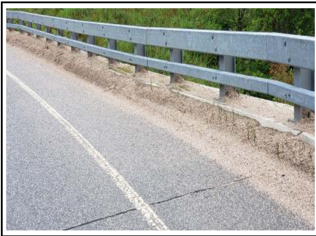
Photo 9 Debris accumulation noted at the edge and over the traffic barrier
