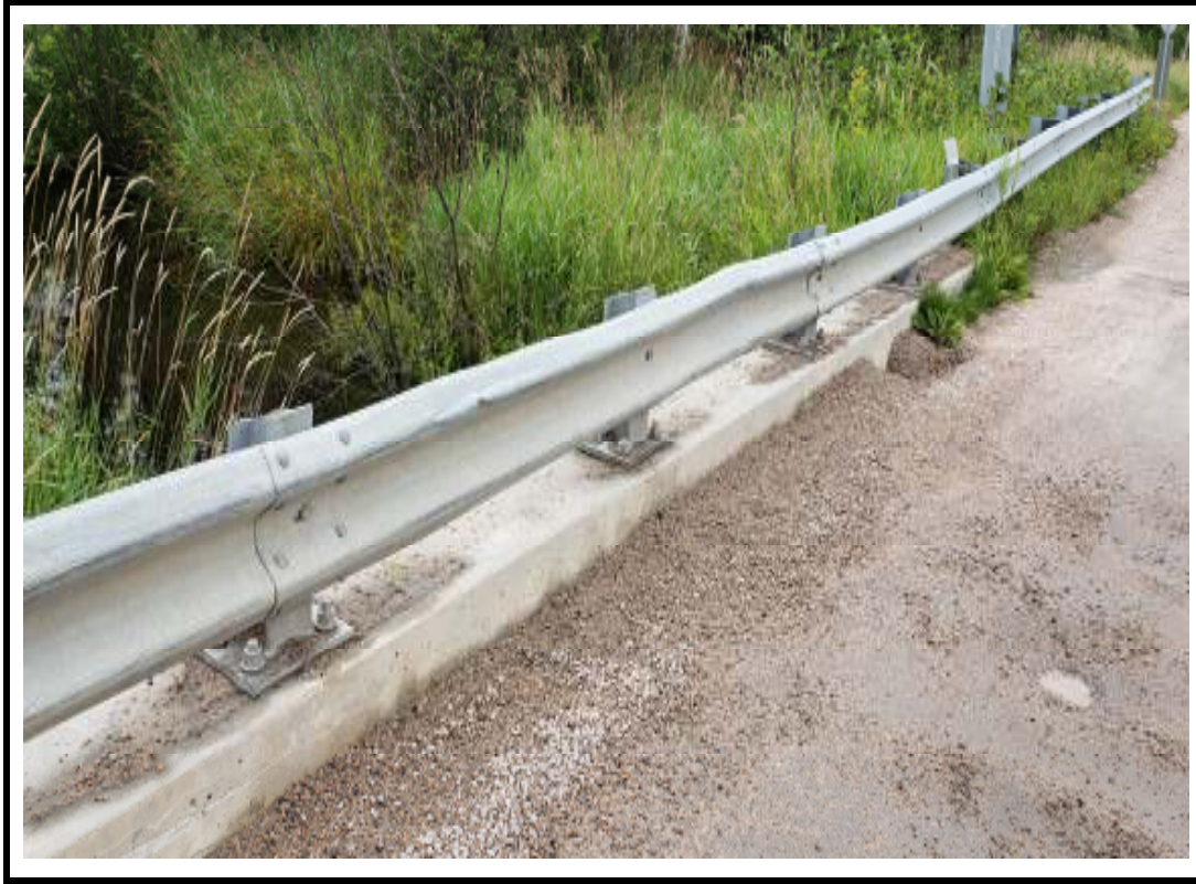
Photo 9 Collision damage noted on north deck barrier
