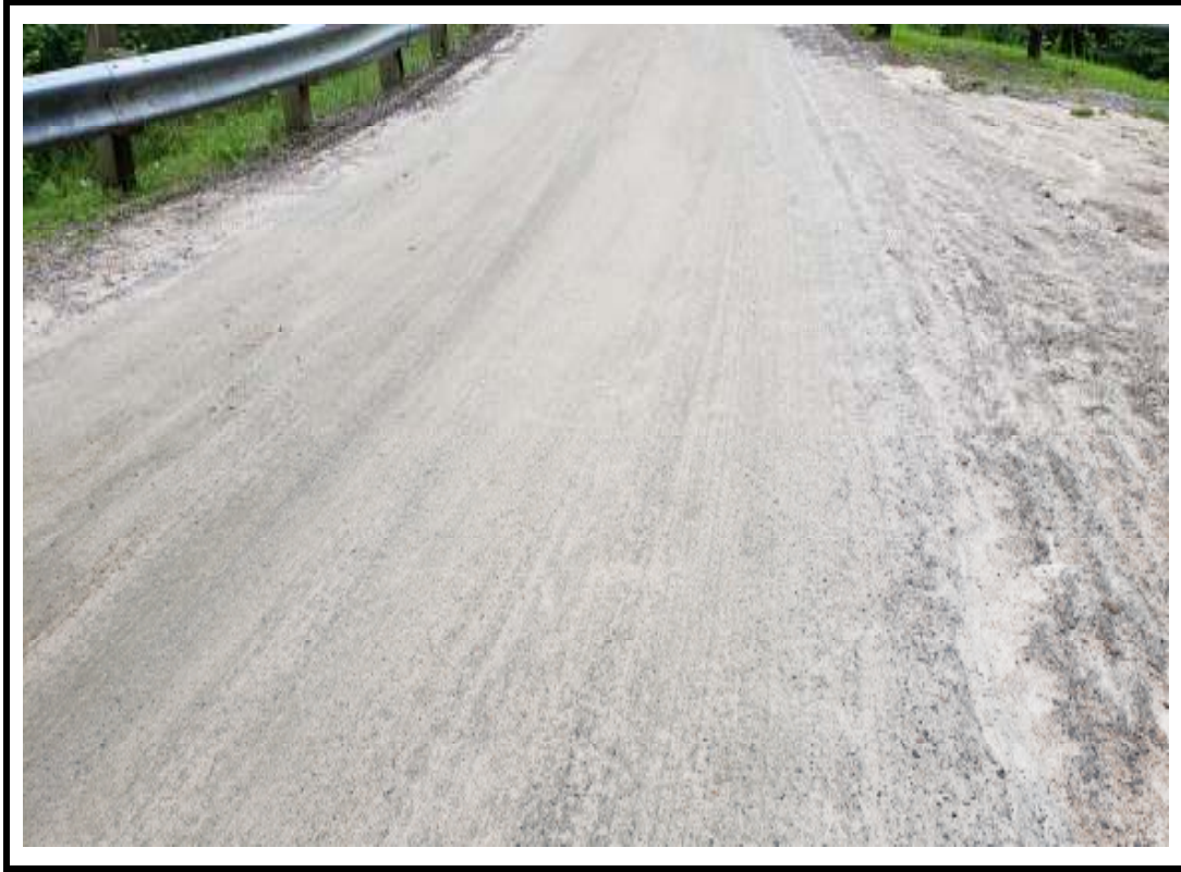
Photo 7 Tire rutting and small potholes noted on approach wearing surface
