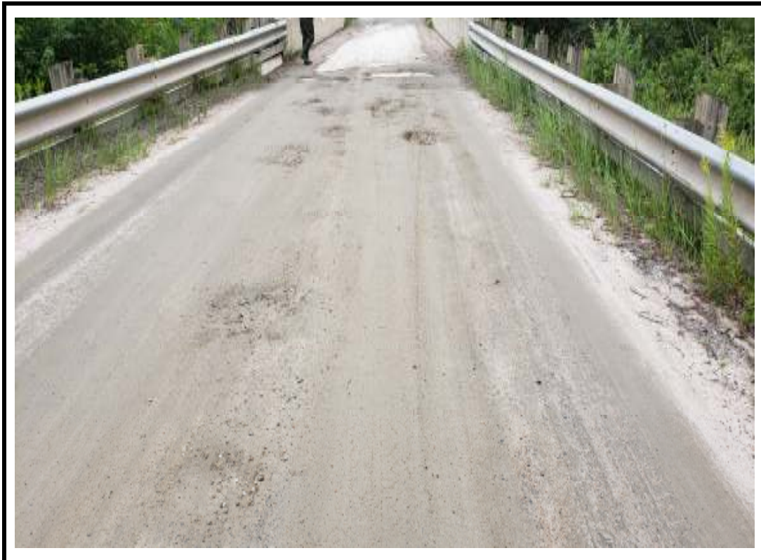
Photo 8 Large potholes and tire rutting noted on approach wearing surface
