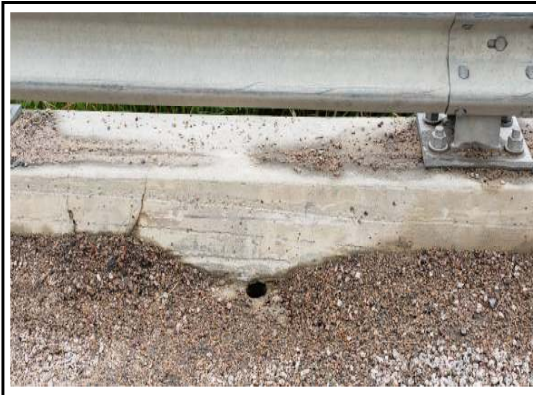
Photo 10 Snowplow damage with narrow cracks noted on curb
