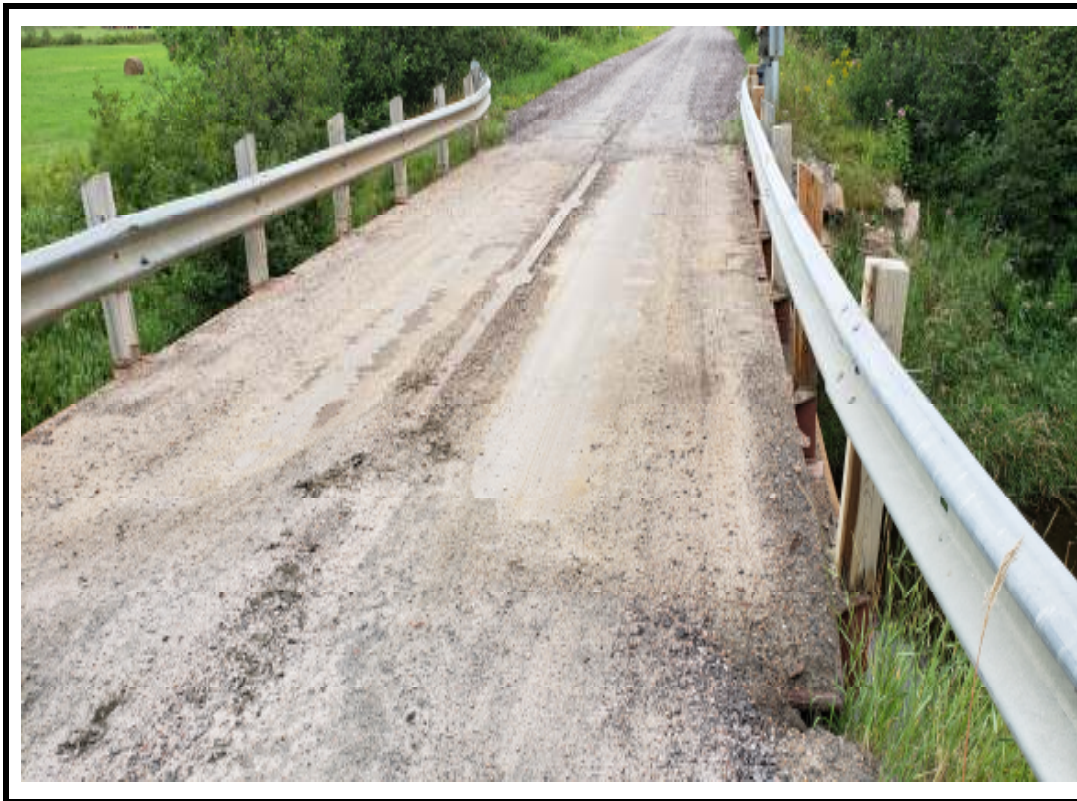
Photo 11 Gravel accumulation noted at center and edge of deck wearing surface
