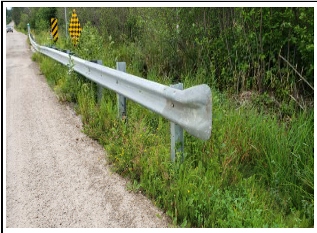
Photo 8 Substandard end treatment noted on southwest corner
