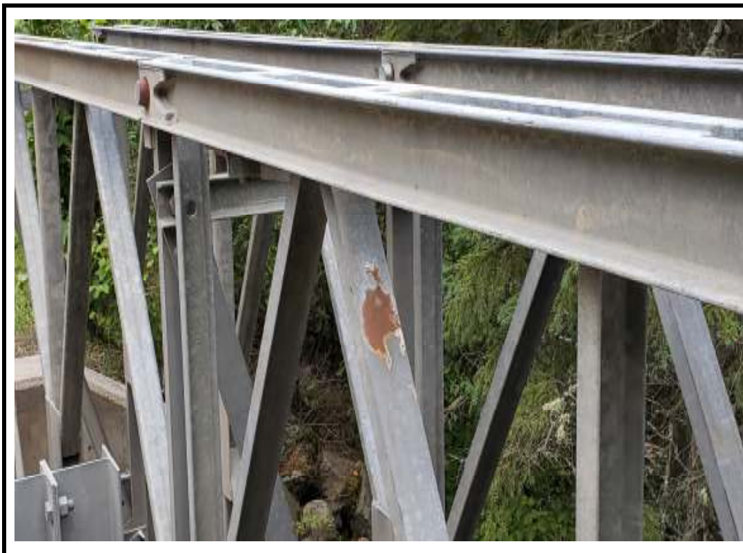
Photo 12 Corrosion noted on diagonal member of bailey panel on bridge barrier
