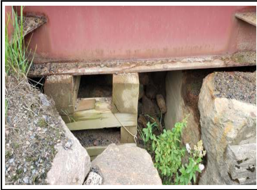
Photo 13 Cracks noted on wooden crib at northeast corner
