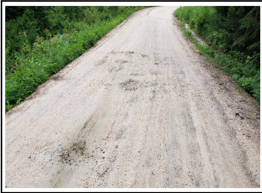
Photo 7 Potholes and loose gravel noted on wearing surface
