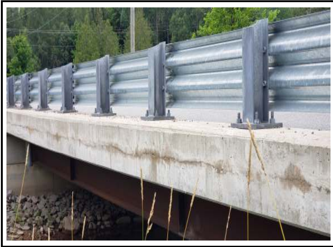
Photo 11 Longitudinal narrow racks with damp stains noted on west fascia
