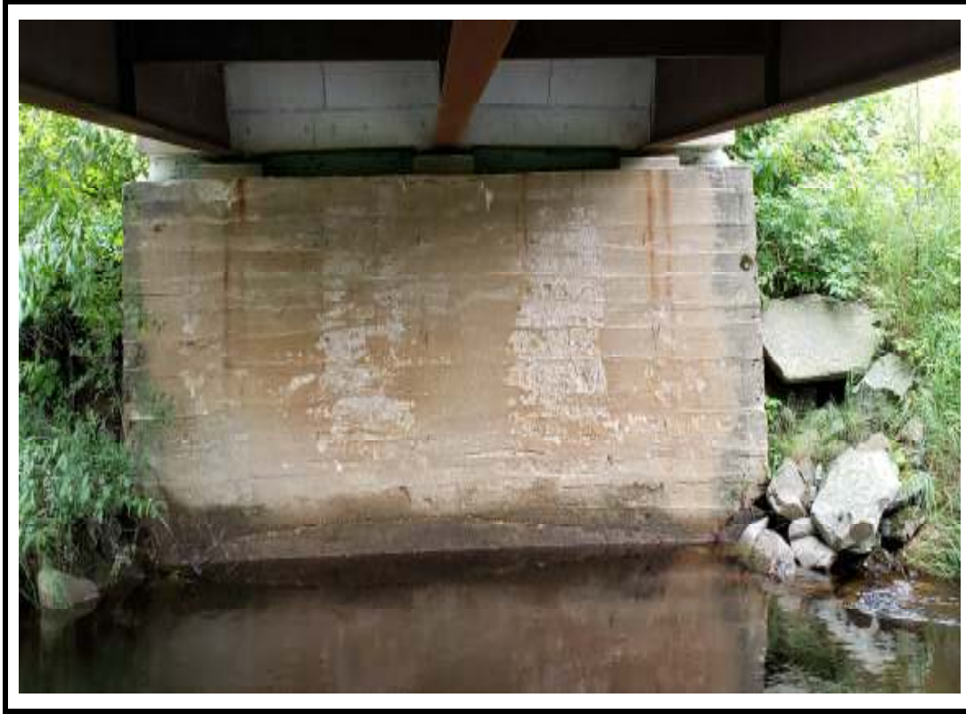
Photo 15 Moderate scaling, honeycombing and spall noted on south abutment wall
