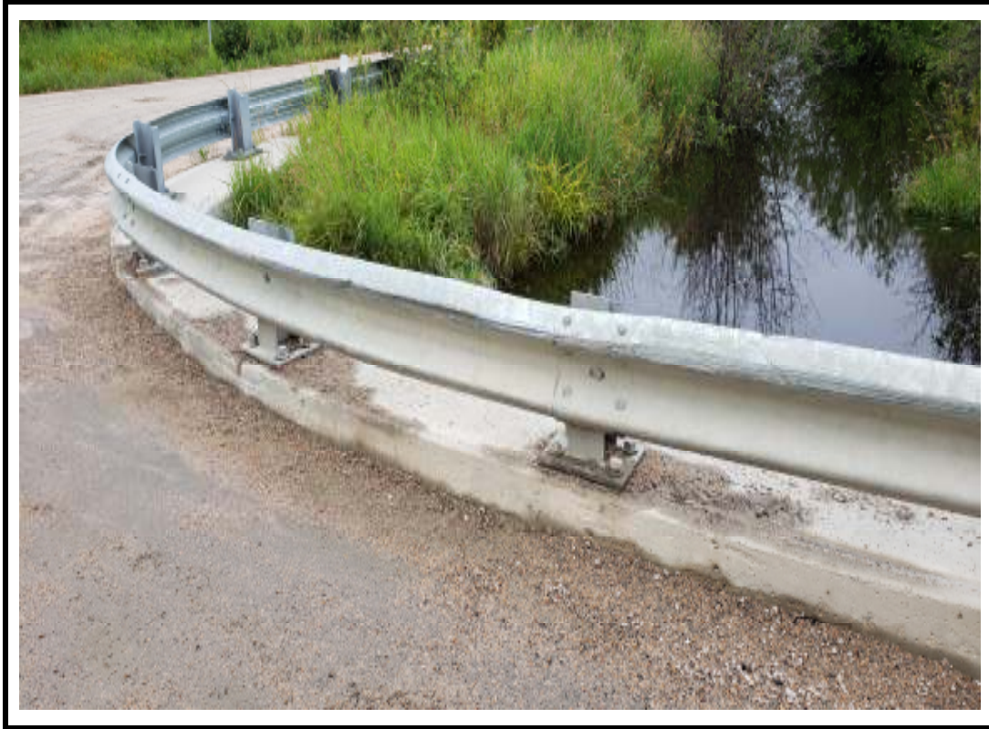
Photo 11 Gravel accumulation noted at the edge of wearing surface
