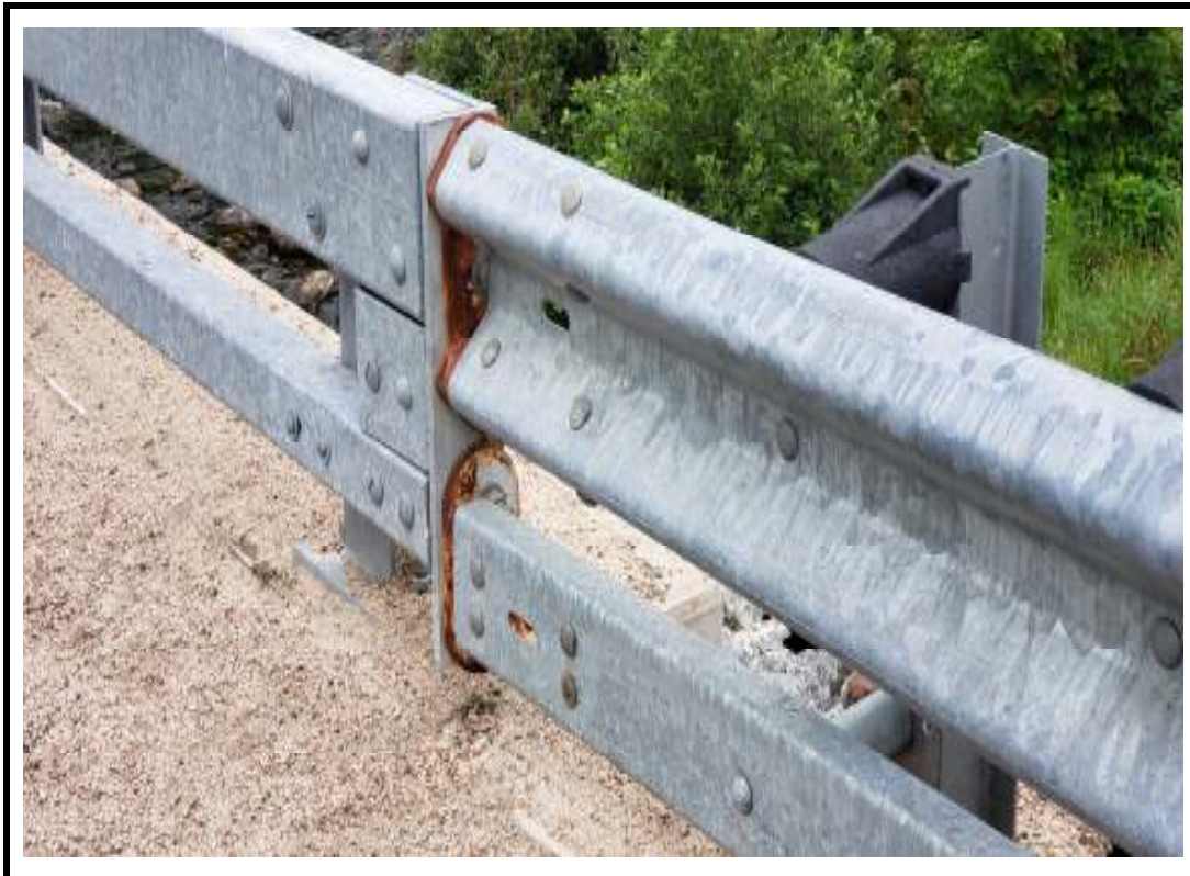
Photo 8 Corrosion noted at connection between approach barrier and traffic barrier
