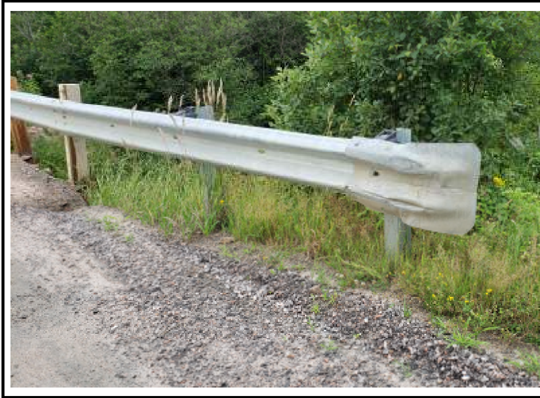
Photo 9 Collision damage on substandard end treatment on southwest corner
