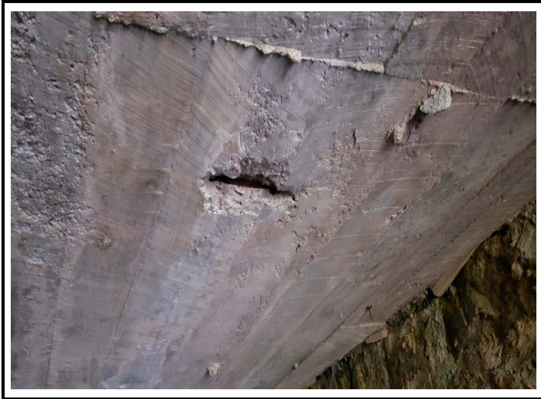
Photo 11 Spalls with exposed corroded reinforcement noted on soffit
