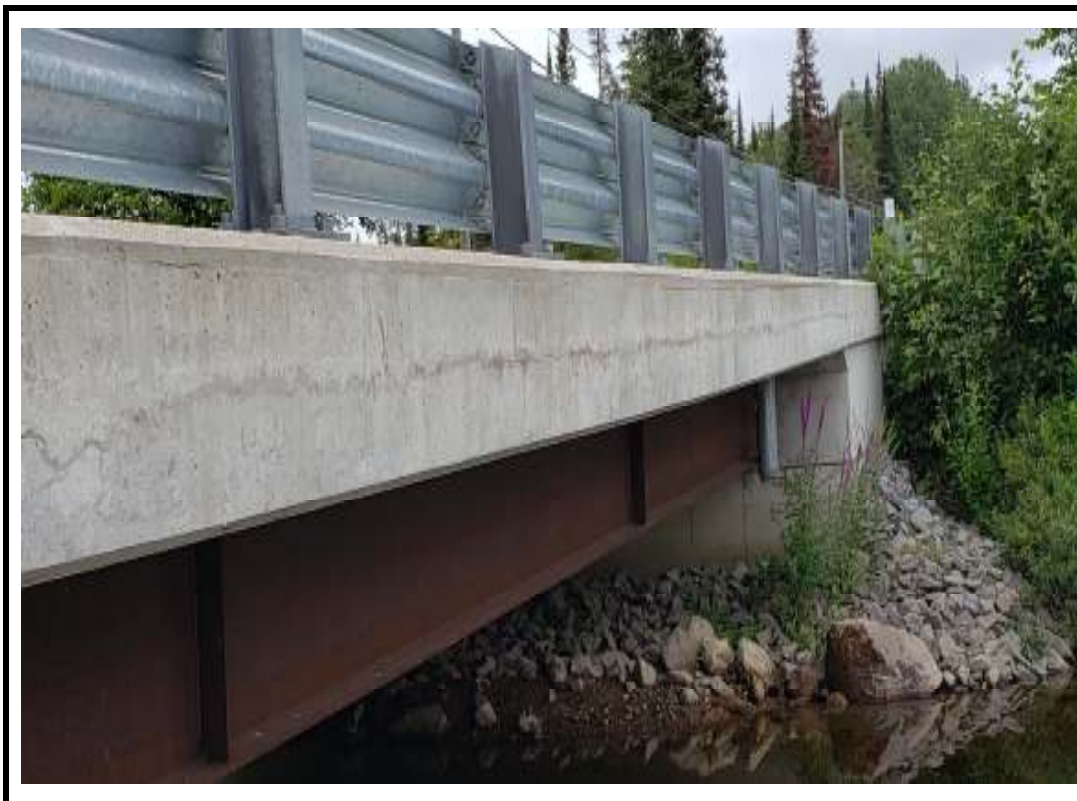
Photo 10 Narrow cracks and scaling noted on east fascia
