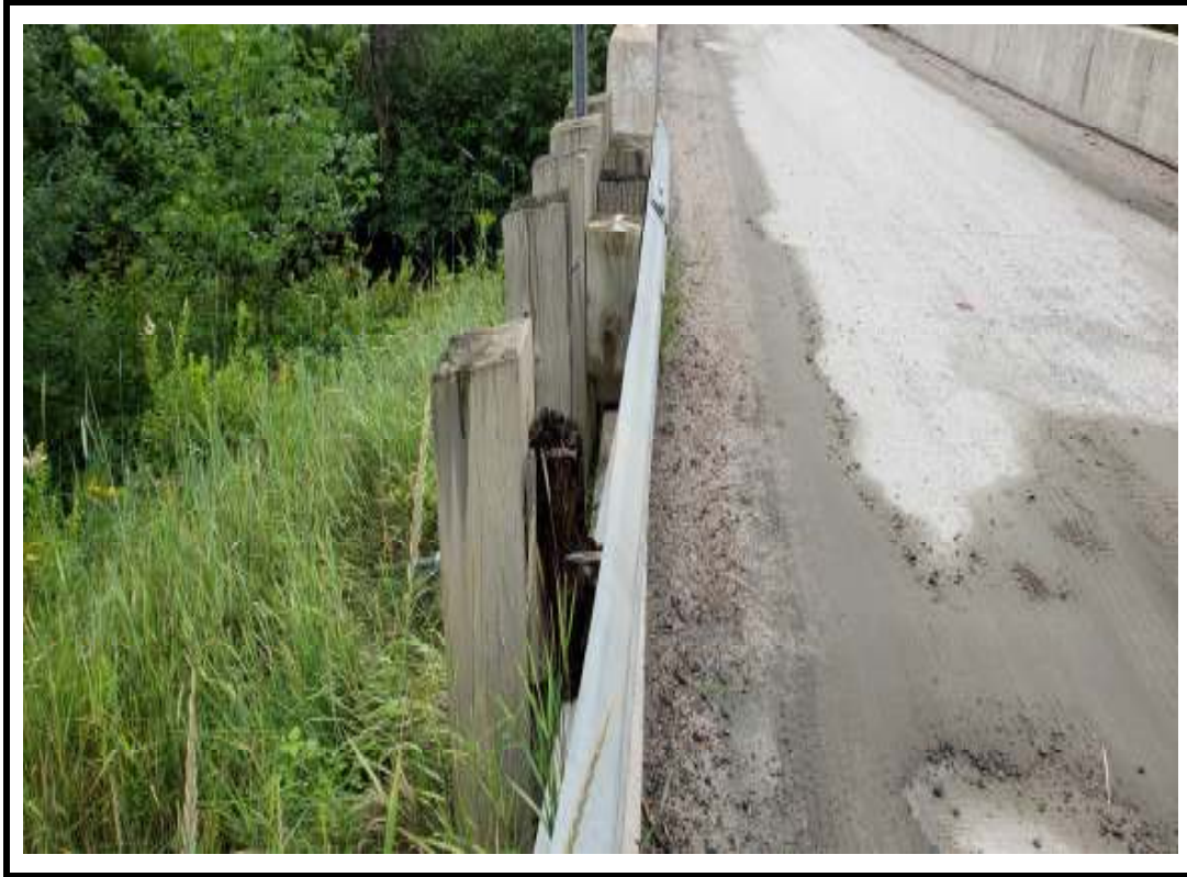
Photo 9 Spacer connected with approach barrier at northeast completely weathered
