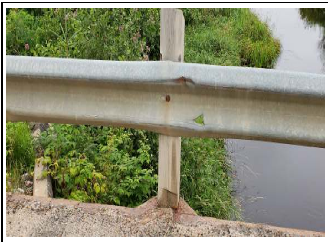
Photo 10 Corrosion and perforation noted on deck barrier
