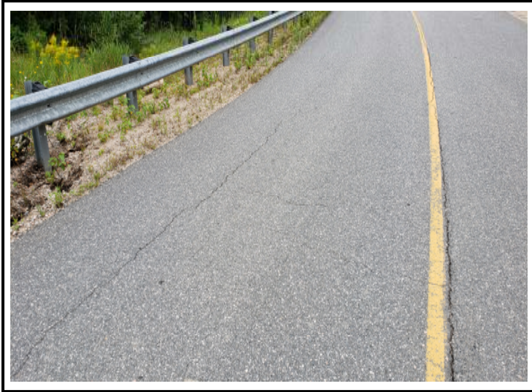
Photo 7 Vertical cracks noted along centerline and edges of approach wearing surface
