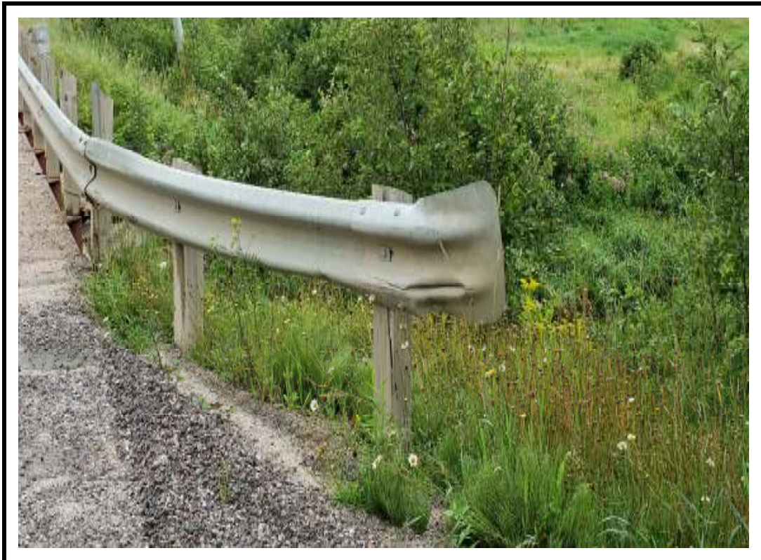
Photo 8 Collision damage noted on northeast end treatment
