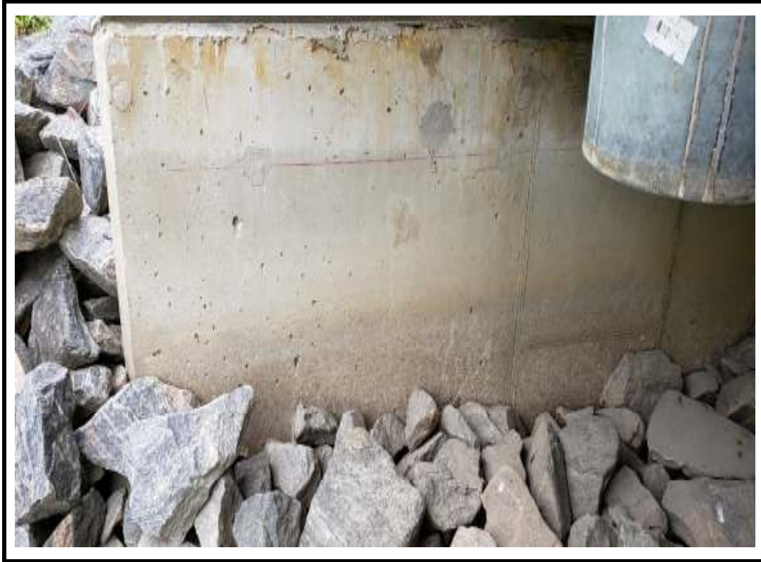
Photo 13 Concrete disintegration and scaling noted on abutment wall
