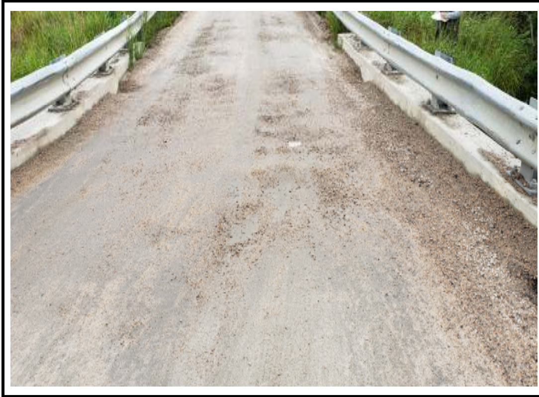
Photo 7 Potholes and loose gravel noted on deck wearing surface
